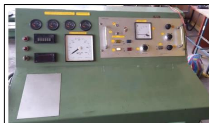
Figura 17–3: Panel de control
